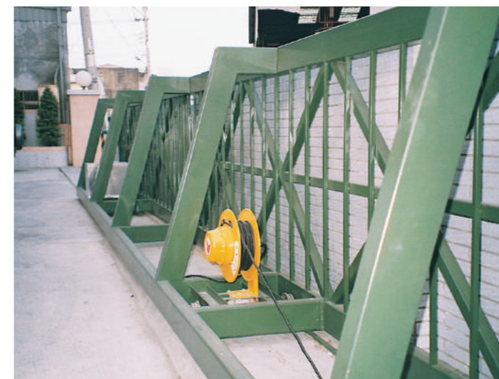
For Gate Door Opening
