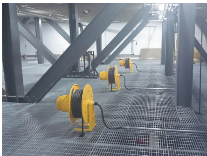
Da Dong Art Center: Power Supply for Stage
